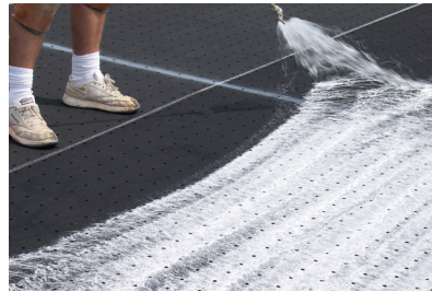
The second picture shows the adhesive being sprayed on a porous pad with holes drilled through for drainage. Note also, in the picture the spider-web pattern of the adhesive being sprayed.
