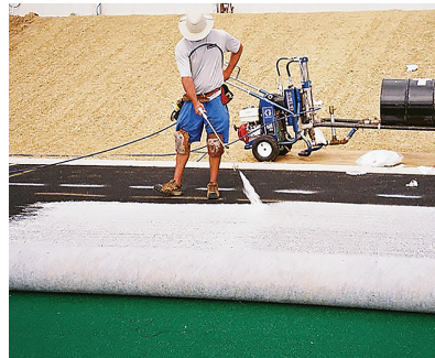
The type of spray rig that is frequently used to install these types of fields. Note that the 55-gal. drum is mounted on a portable carriage, along with the airless spray unit, so that the adhesive can be moved as the job progresses without any great effort. It also shows the adhesive being applied.
