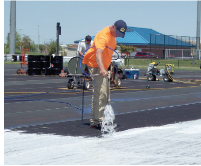
The first and perhaps the most important picture is the one showing the adhesive being sprayed with a spider-web pattern. Note also in the picture that the black sub-surface telegraphs through the white-sprayed adhesive indicating there are numerous places for the water to penetrate through.
